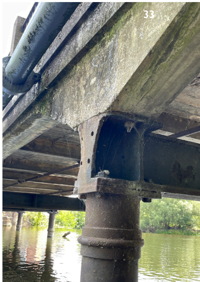
33. Tapered end of cast-iron beam, with four holes for dowels, missing end cap (upstream face - Pier 4) - 8.8.25.
